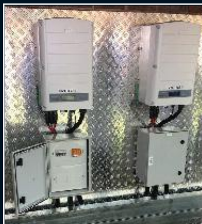
Combiner Boxes for PV systems
